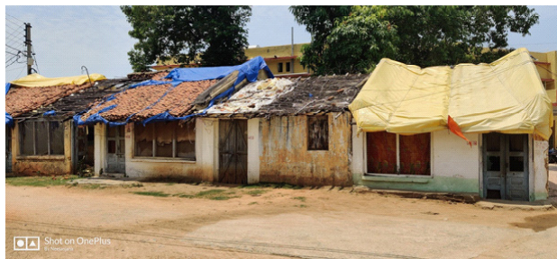
Staff quarters at CHC facility (Currently quarters are not being used because the roof had fallen down)
