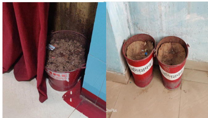
Sand buckets not in usable condition at District Hospital
